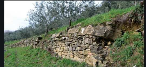
2 - A greater part of terrace dry stone walls in Krvavce have collapsed
