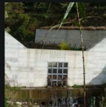
10 - Vernazza, concrete embankment to be fixed
