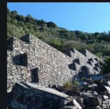
13 - Vernazza, stone filled cages to prevent landslides to hit on a path
